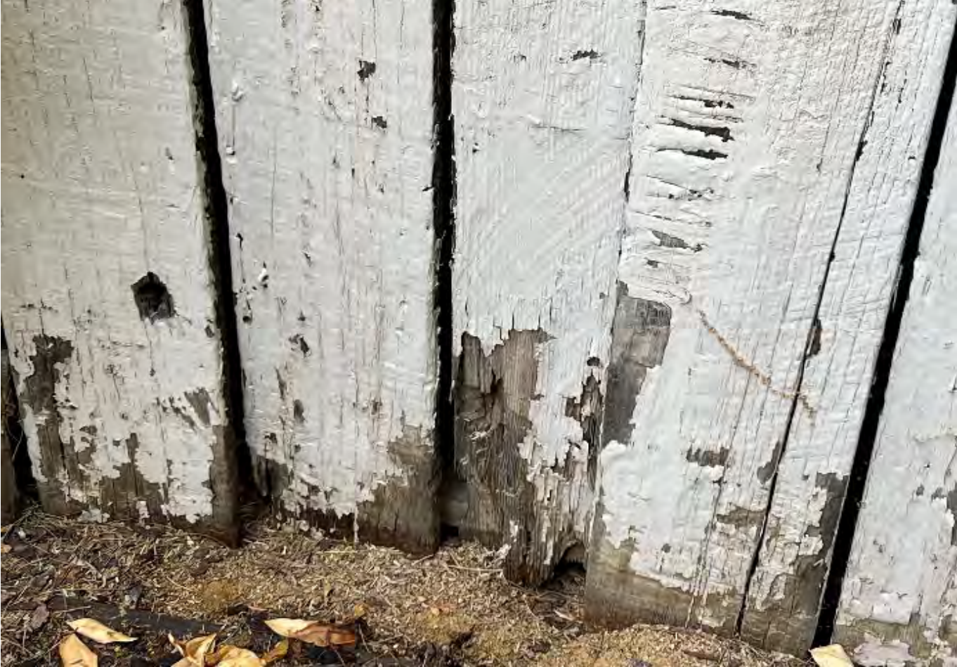
Alternate view of east(side) wall deterioration
