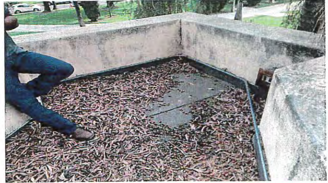
The building has a built-up roof with counter flashing and conduit that runs along the flashing. It is recommended that the conduit be removed if not operational and reinforce the existing roof with WeatherWeld.
