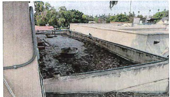
All vents and piping support penetrations should be sealed during roof work or removed if not being used.
