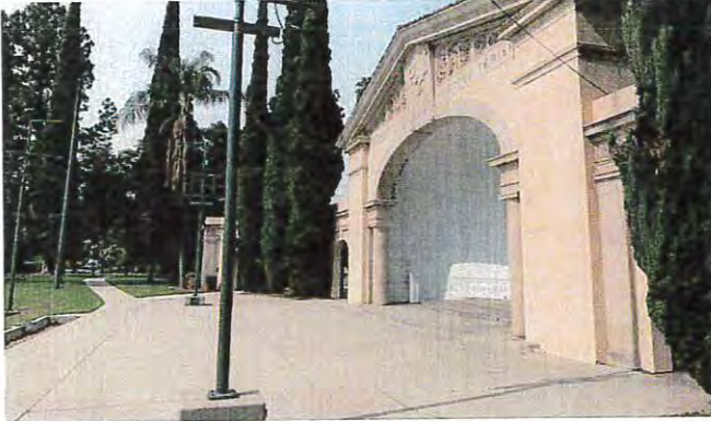
The City of Redlands building is a historical building with a roof that has reached to end of its ability to keep the building watertight.
